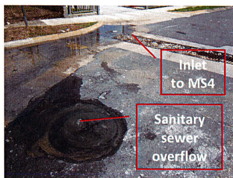
Wastewater flowing from a sanitary sewer access manhole to a nearby storm drain system inlet. Photo: PG Environmental
